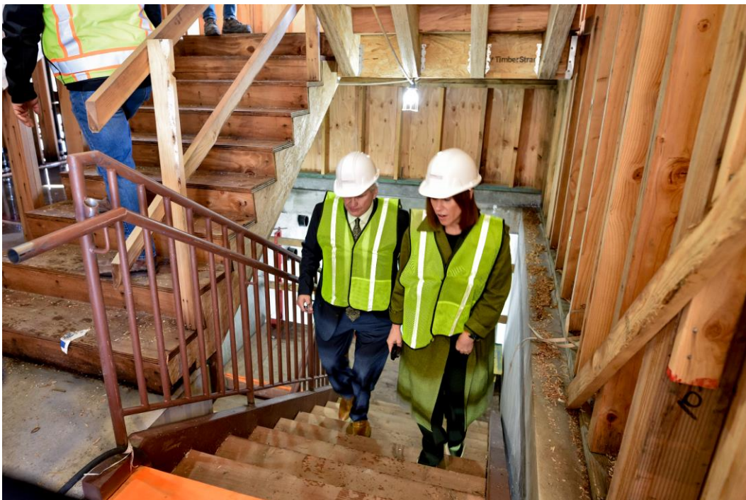
HUD Principal Deputy Assistant Secretary Richard Monocchio (left) and Santa Clara County Housing Authority's Director of Real Estate, Flaherty Ward tour the construction site of Bellarmino Place.
